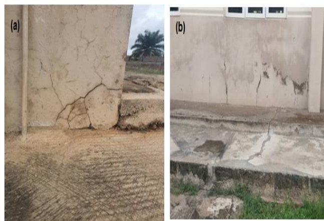
Plate 1. Symptoms of Distress observed on the building. (a) Basal Mesh of Cracks (b) Rising damp, blistered paint and flaked plaster.
